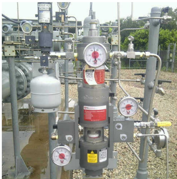
Figure 8 – VPC Replaces Existing Becker VRP VRG Controls shown above replaced Dresser VRP Controller to provide improved control and greater durability in aggressive environments.
