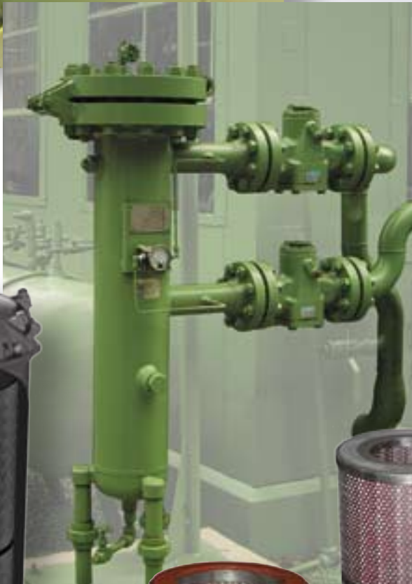
This Sparks™ coalescing filter is used for its combustion fuel.
