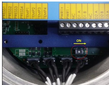
Figure 5-1 - Line termination resistor switch
